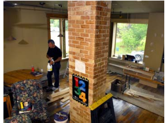
Robert Wilson/Record staff The REEP House is a century-old Kitchener house with green upgrades.
